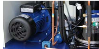
Pump P3 (3 barg) / P5 pump (5 barg, optional).
